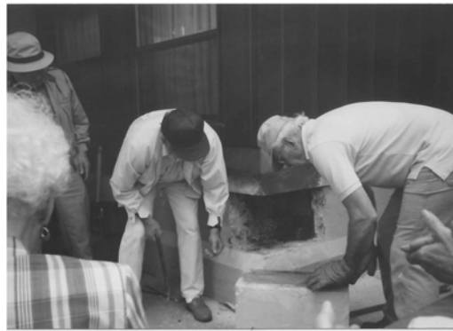
Removal of the 1936 cornerstone. Unfortunately the contents inside were too damaged by leaking water and old age.
